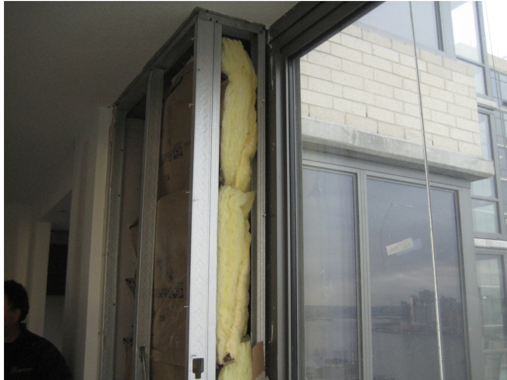
Spandrel area with insulation tight up against #4 surface of insulating glass
